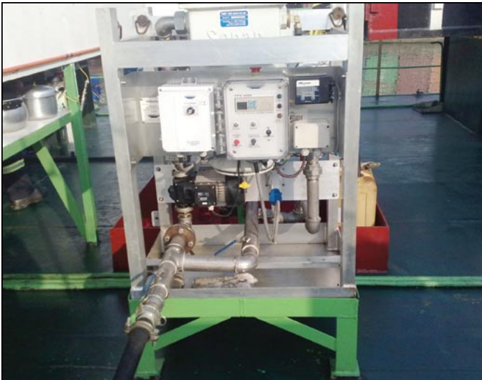
Fuel Polishing System installed on dredging barge.
