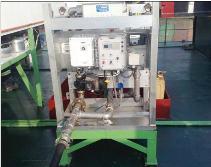
Fuel Polishing System installed on dredging barge.
